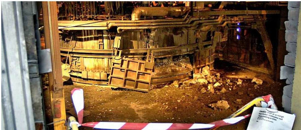
Figure 3. Photograph showing structural damage suffered by Elkem Thamshavn silicon furnace in 2006 water-metal explosion, which resulted in 1 fatality. Photograph by S. Fugelsøy [8].
